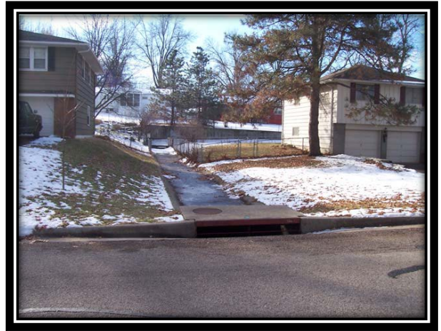
Example of an overflow drainage problem well upstream from the mapped Special Flood Hazard Area – the structure on the right is at increased flood risk due to “overflow” water from the storm sewer entering through the garage doors.
