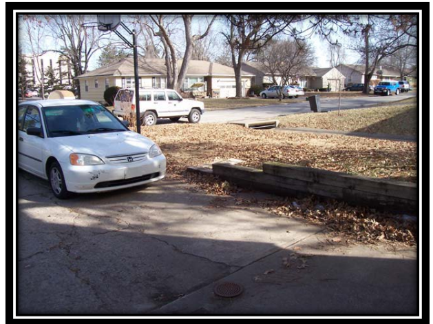
In another view of the same property, notice the retaining wall constructed by the property owner in an attempt to direct storm drainage overflows away from the garage. The property owner volunteered information that was invaluable in determining the exact cause of flooding.
