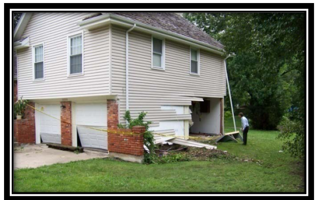
House damaged by flash flood in June 2010. This house is just upstream from a repetitive loss area that is being mitigated by a project to be constructed in 2014.
